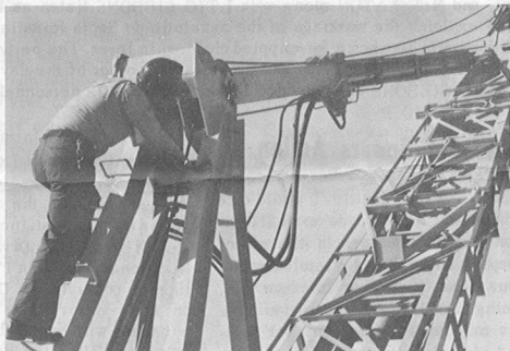
Inspecting the bearings on traveling cranes is a risky business, testifies EN3 ZAGOZAN
