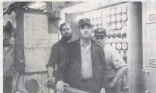
Behind these three men is the control panel where the ship's power is constantly being watched. EMFN A. Stiles, EM1 R. Hatcher, and EM2 C. Coakley are standing the watch.
