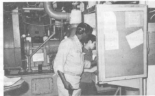
MMC A. Smith checks machinery readings in the engine room with FA W. V. Tangi.
